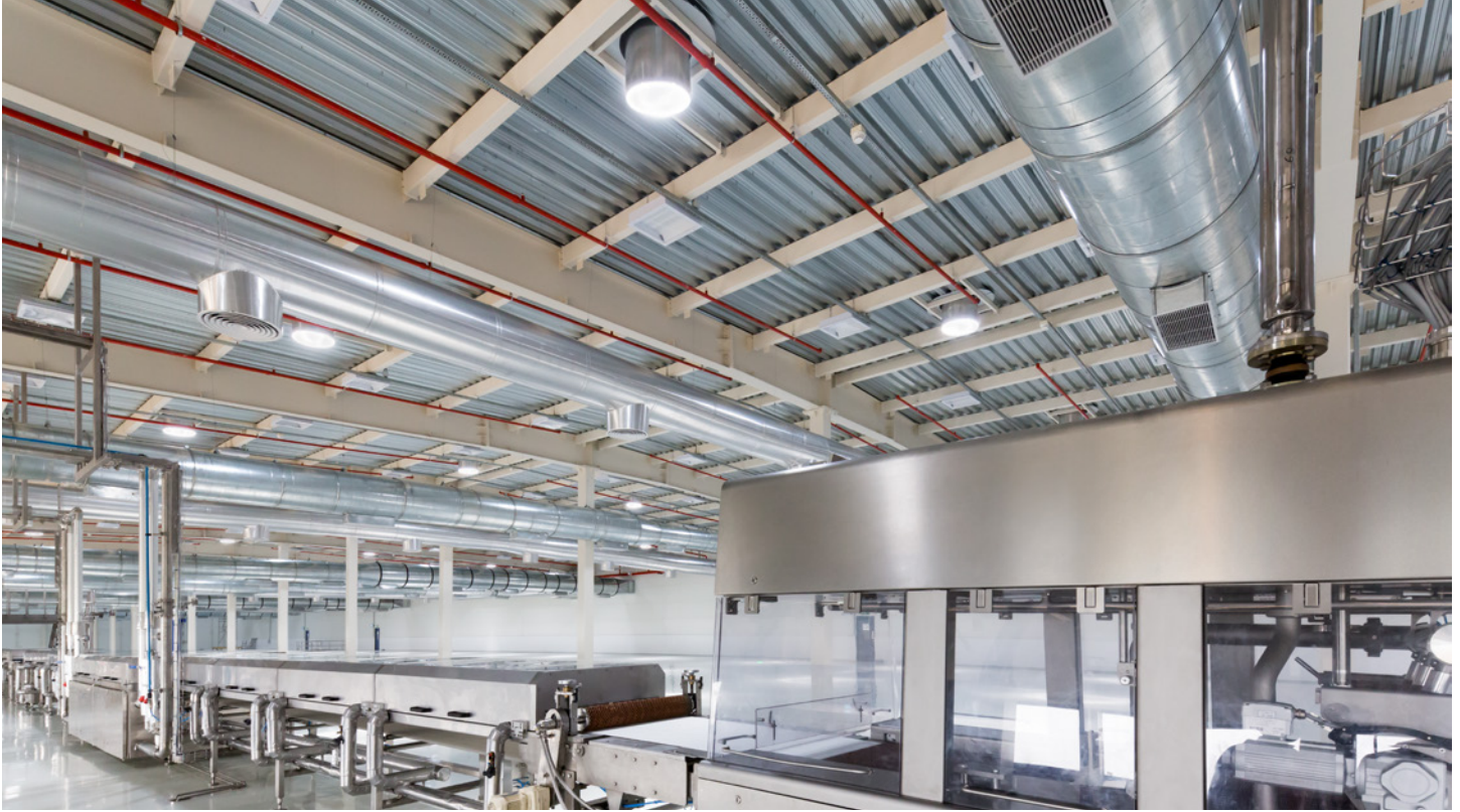
Solatube units deliver bright daylight without solar heat gain to this Mars India production area.
