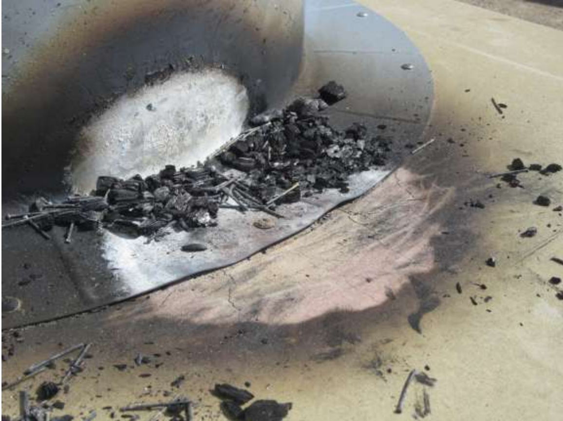
Photo No. 5 Warping of 330 DS Flashing
